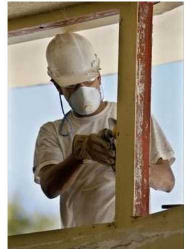
The Ledger/Pierre DuCharme Augustine Campos, with Henkelman Construction, Inc., sands off old paint from a window frame in the Frank Lloyd Wright designed Fletcher Theatre on the campus of Florida Southern College in Lakeland, Florida February 16, 2009.
