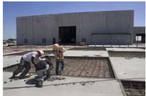
MICHAEL WILSON | THE LEDGER CONSTRUCTION WORKERS are finishing the new Ring Power Corp. facility near the intersection of the Polk Parkway and U.S. 98 South in Lakeland.
