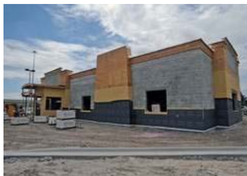
SCOTT WHEELER / THE LEDGER LONGHORN STEAKHOUSE is being constructed in North Lakeland, with an expected opening date at the end of the year.
